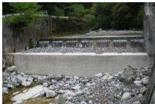
Stream Intake Works in normal time
